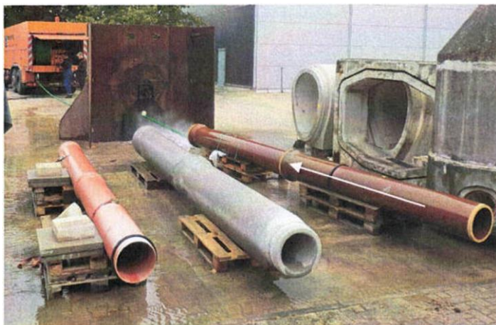
Figure 5: Trial implementation test segment 1 (direction of flush in the direction of the arrow)
